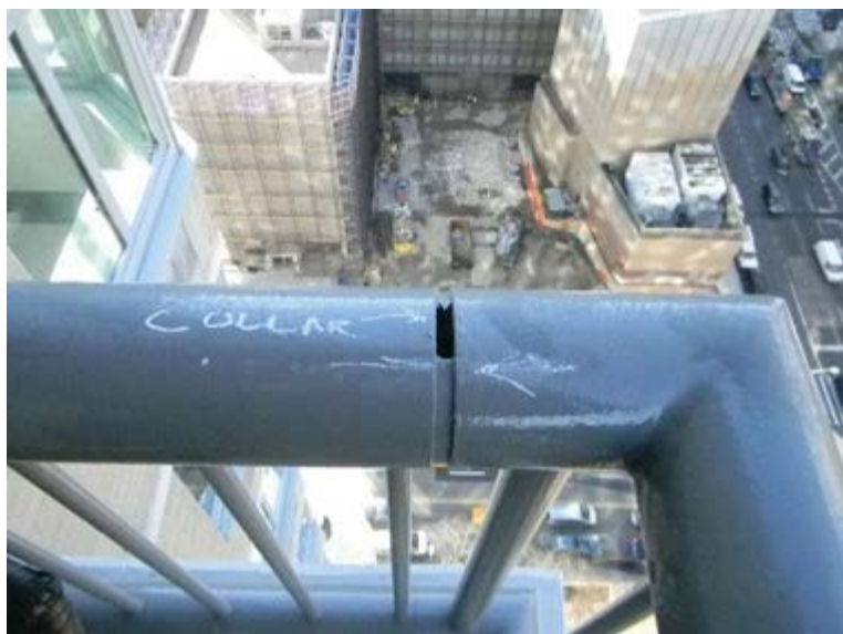
Typical balcony railing deficiency
